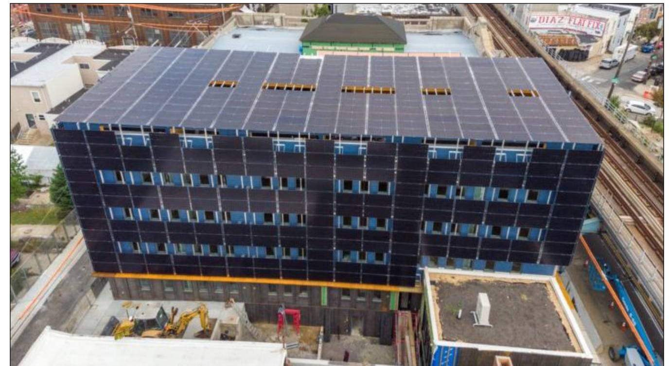
Philadelphia design-build architecture firm Onion Flats installed a 176-kW solar system with a rooftop canopy and wraps around the east-, west- and south-facing walls of its Front Flats apartment building. Source: Onion Flats
